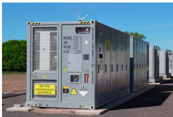
Battery energy storage systems
